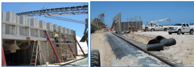
Salt vaults at Shark Bay Resources
